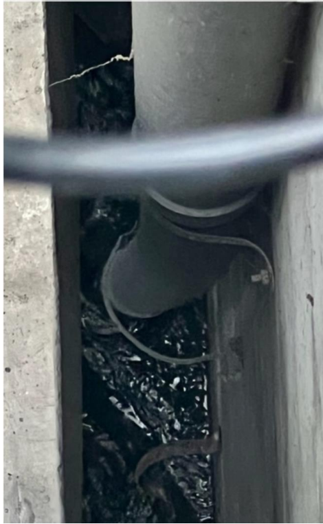
Figure 1: Image of broken NFL channel sensor housing
